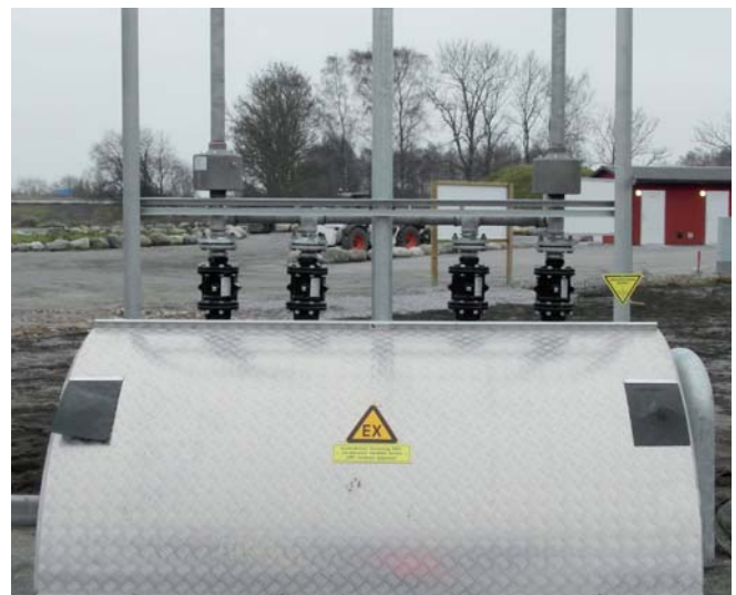
Example of Servus installation at the ventilation stack.
